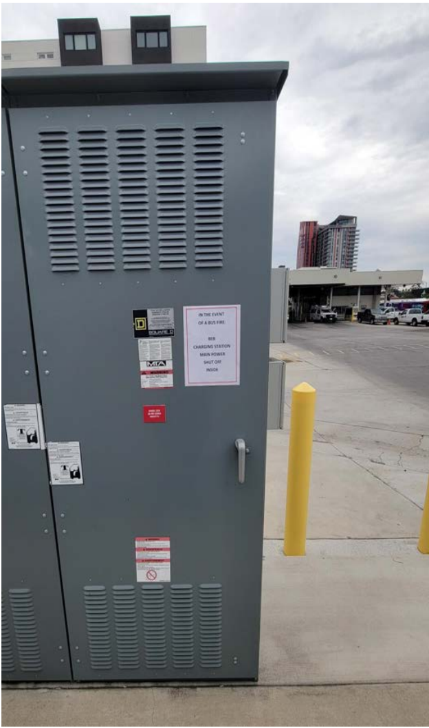
Figure 1.1 Breaker box exterior Figure 1.2 Breaker box interior
